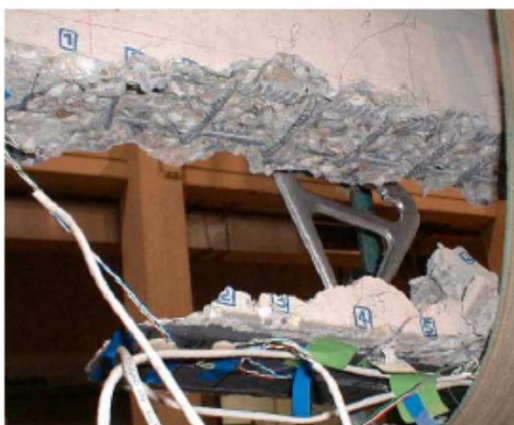
Type 2: at internal steel reinforcement level
